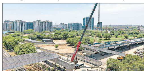
The 650-metre-long bridge is coming up at an estimated cost of Rs 75 crore. EXPRESS
